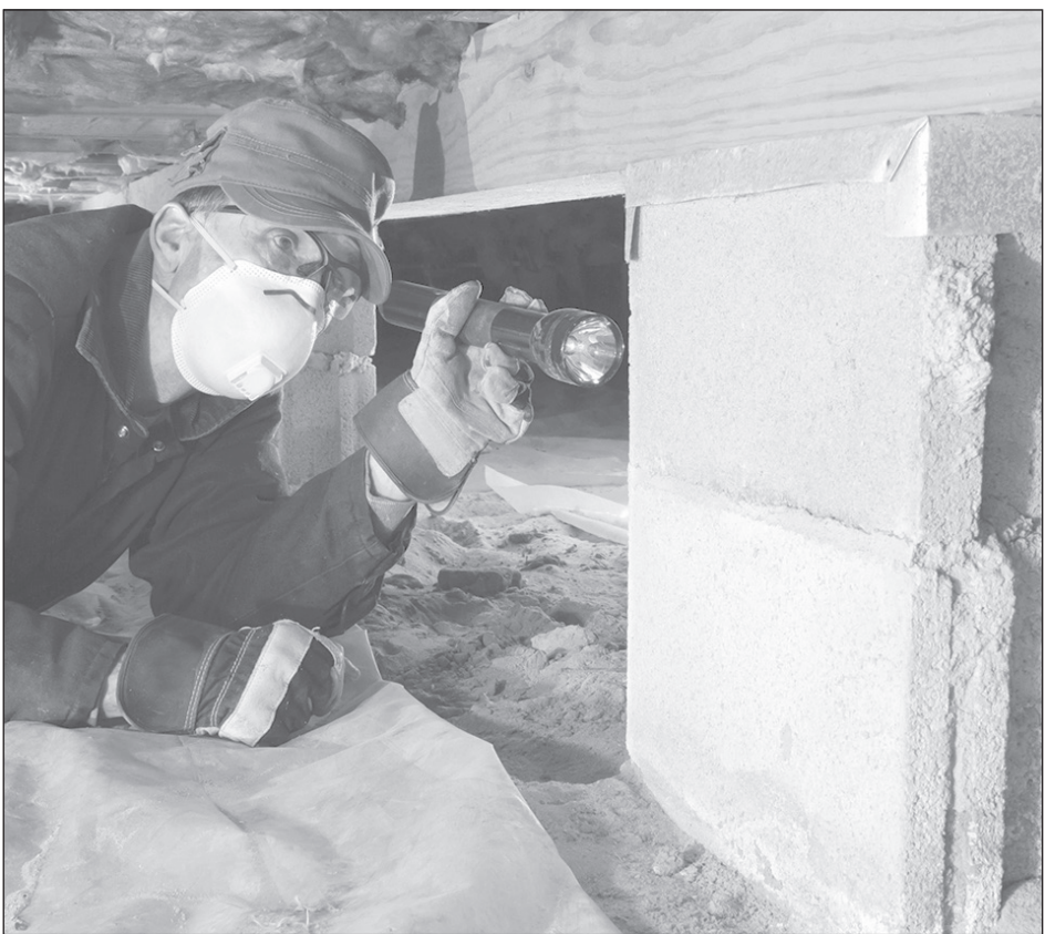
Contributed photo Foundation issues are a component of home ownership that can be easy to forget, as such concerns are not necessarily evident in frequently visited areas of a home. A foundation provides structural integrity for the entire home, so addressing damage is essential.
